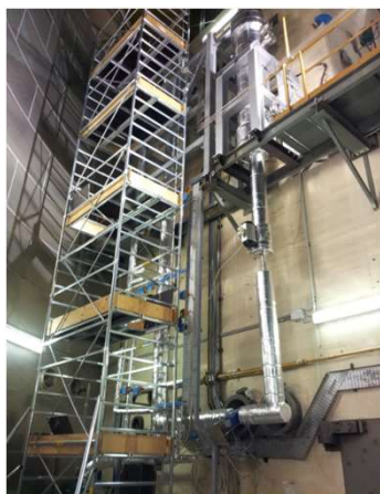
HELENA loop type facility
